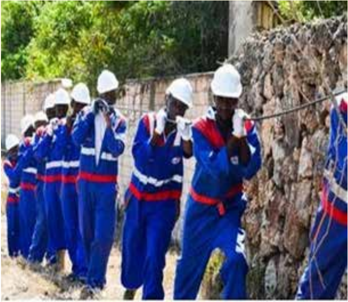
PROJECT: DESIGN, SUPPLY, INSTALLATION AND COMMISSIONING OF ADSS FIBRE OPTIC CABLE ALONG MEDIUM AND LOW VOLTAGE LINES.
